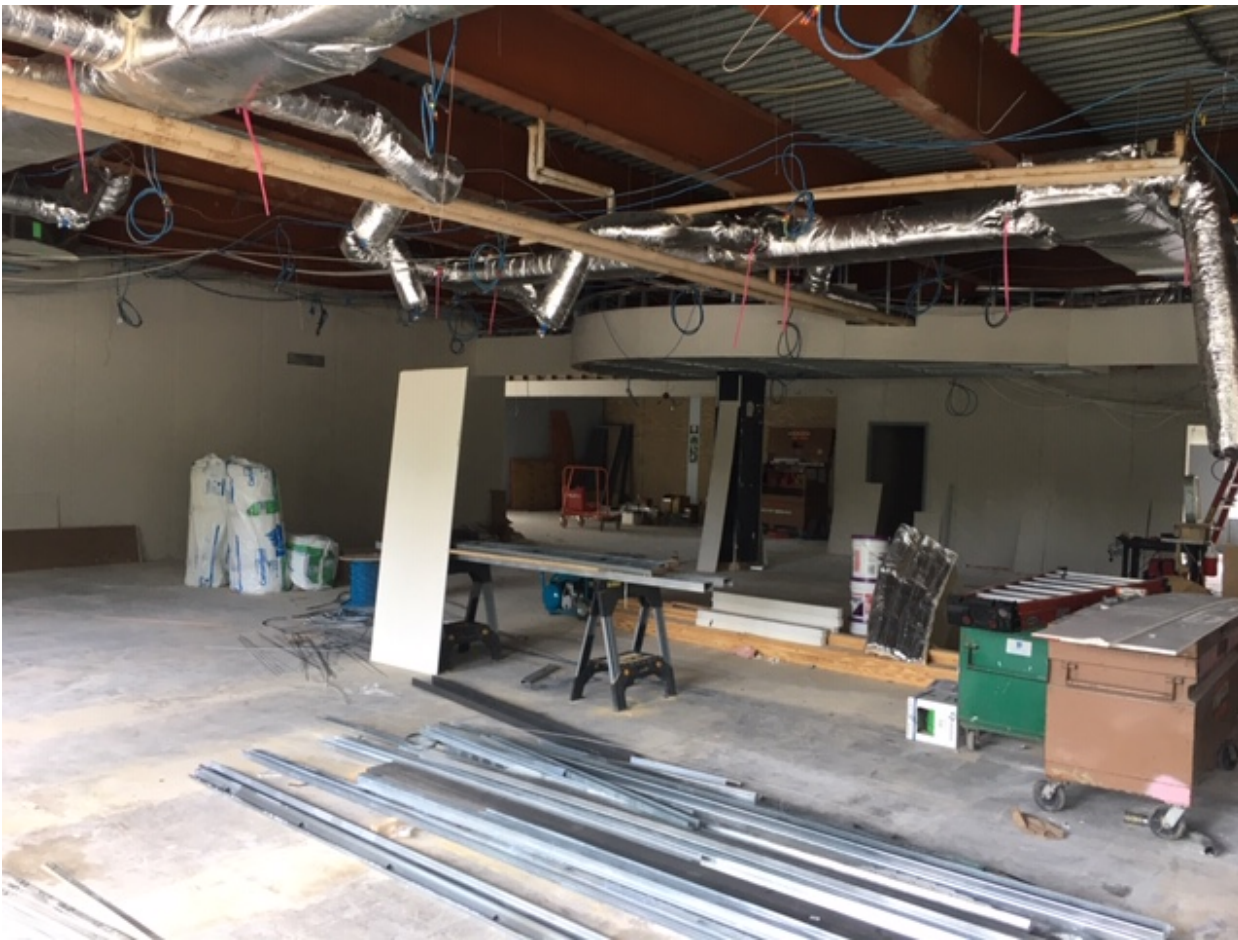
Week 9 – Progress of work in the Library highlighting the curved soffit over where the circulation desk will be.
