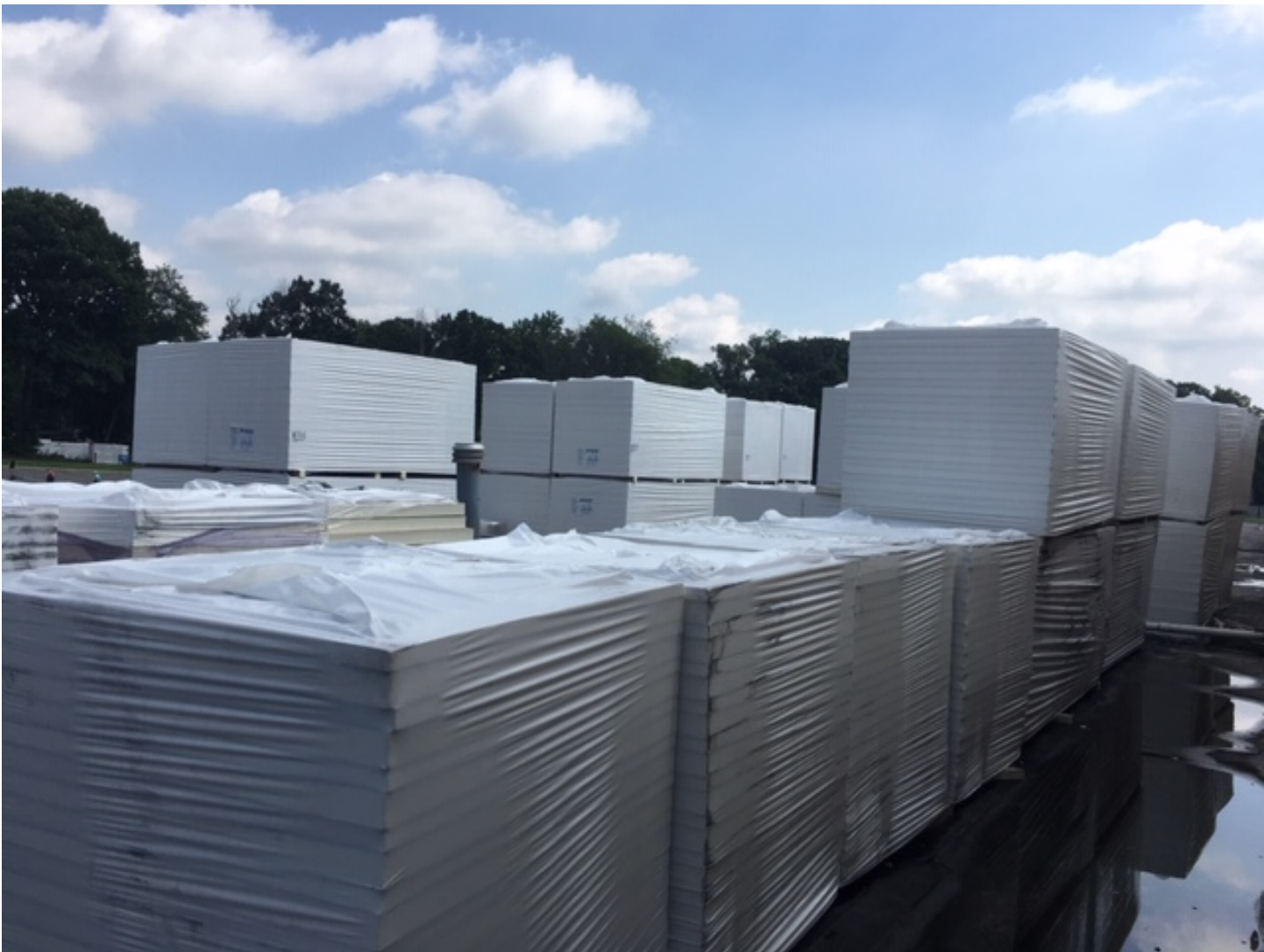
Week 9 – Staging of material for the installation of the new roof assembly over the Locker Rooms
