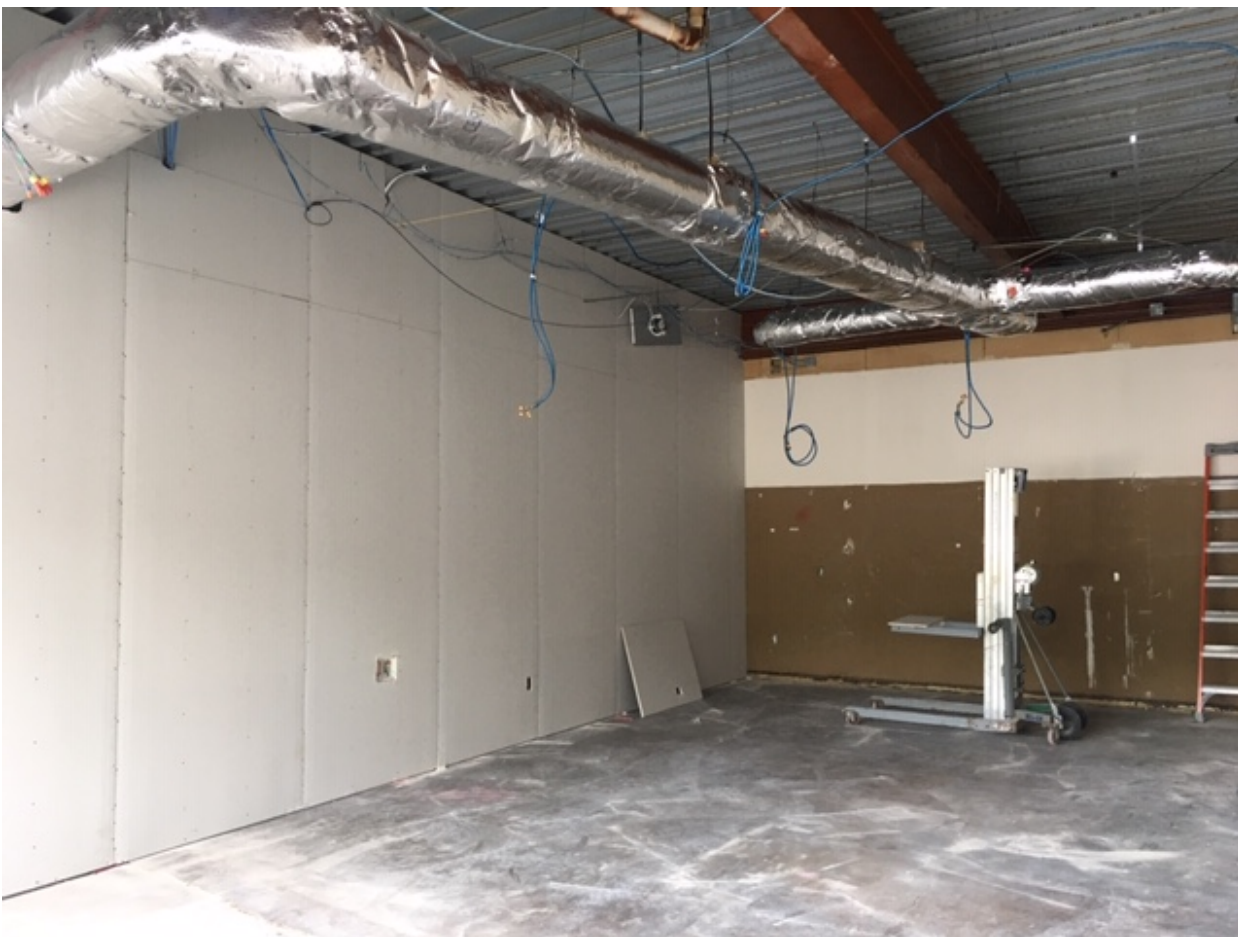
Week 9 – Partition ready for spackle & taping of joints in Math Rooms 331A
