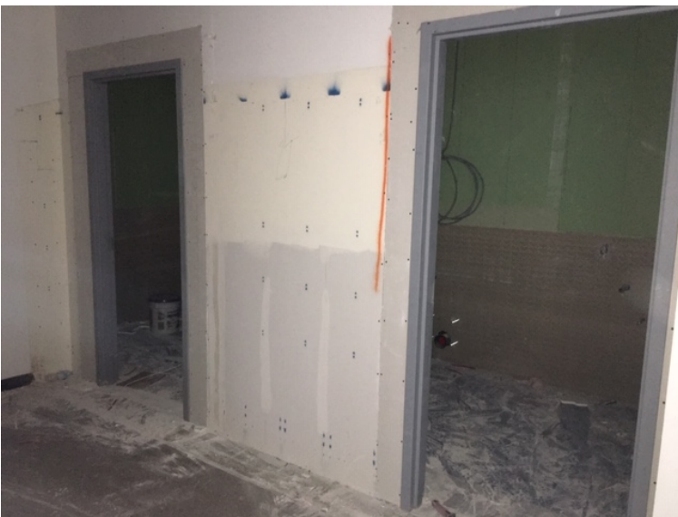
Week 9 – New bathrooms in the Science Wing being prepared for wall finishes
