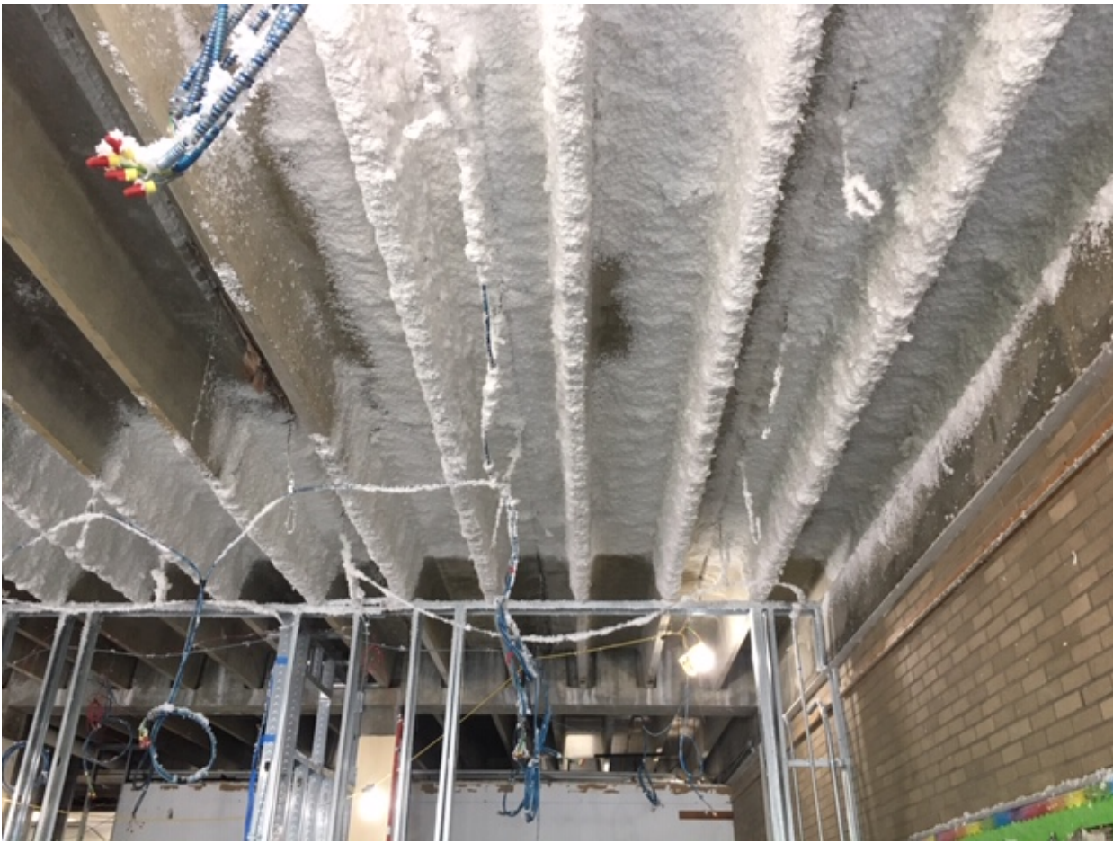
Week 9 – Spraying acoustical foam material onto the underside of the existing deck in the Music Wing
