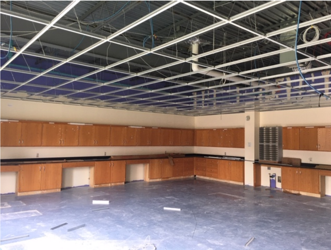
Week 9 – Installing new ceiling grid for support of new ceiling tiles and new light fixtures in an existing Classroom in the Science Wing
